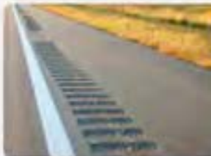
Longitudinal Rumble Strips Photo courtesy of MarekPhotoDesign/Adobe Stock
